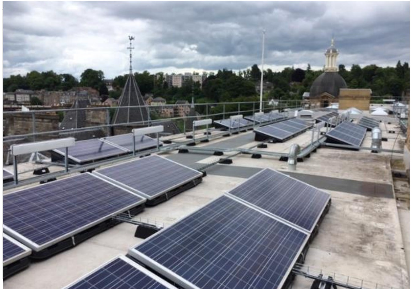
Rooftop PV installation on Perth and Kinross Council's offices in Perth
