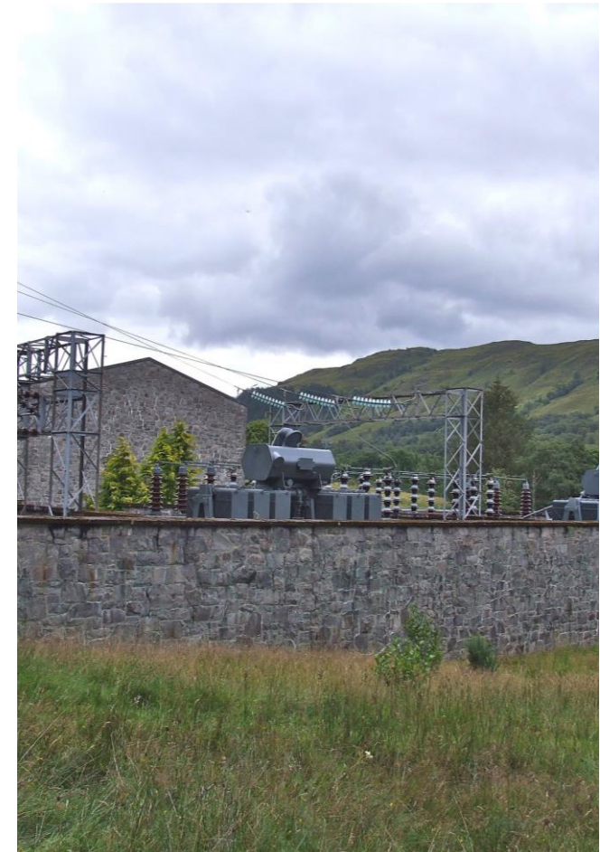
Powerlines in Lochay
